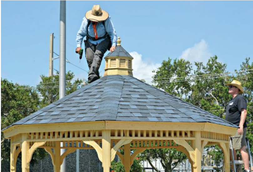
Satellite Beach Lions in Florida worked three weekends building a US$12,000 gazebo for the community as part of a Lions Centennial Community Legacy project. Boy Scouts helped.
